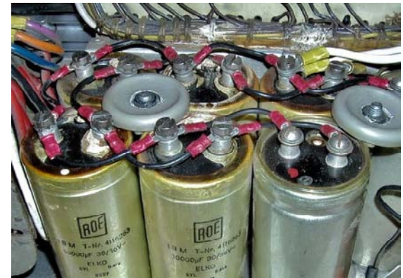
Several leaky capacitors
