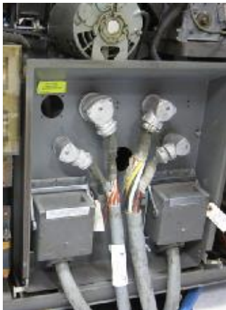
Figure 38: Power and Signal Cables in the 1402
